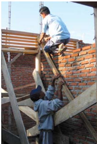
Over the past year, Indonesian families have been constructing new homes with the hope of living in permanent shelter once again.
